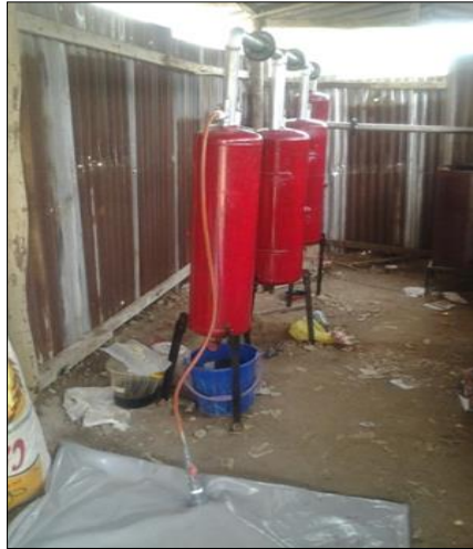
Figure 2a Gas storage bag connected to the gas scrubber (before experiment)
