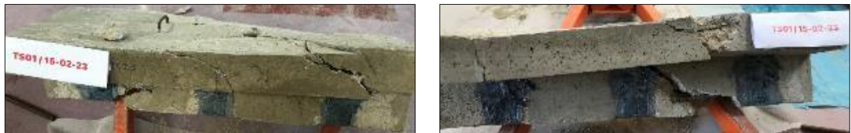
Figure 5 Crack pattern of the sides of the U-jacketed FRP strips at strengthened beam TS01
