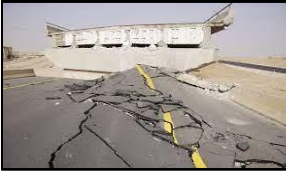
Figure 7 Weather effect on the bridge
