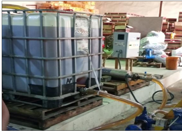
Figure 1 Process setup of the ultrasonic processor at Techno Oil facility
