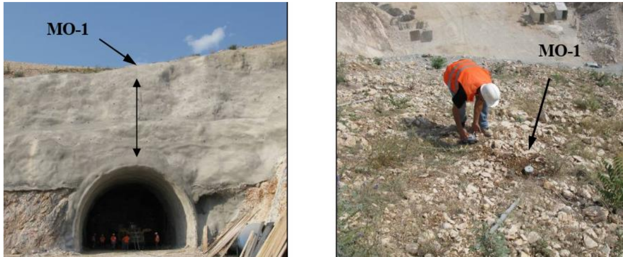
Figure 6 Location of observation site and measurement of peak oscillation speeds in relation to the blasting area
