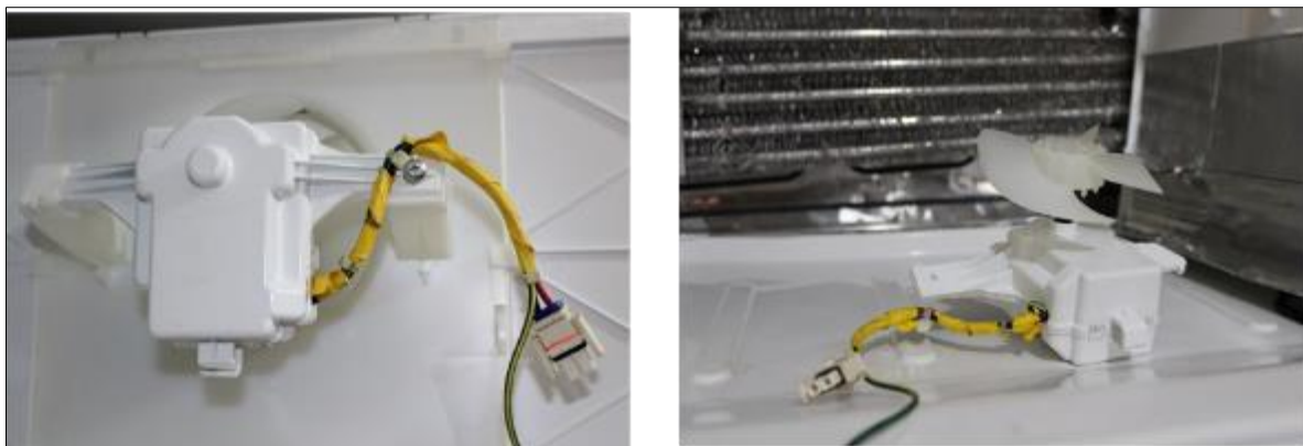
Figure 4 Refrigerator fan B and fault simulation
