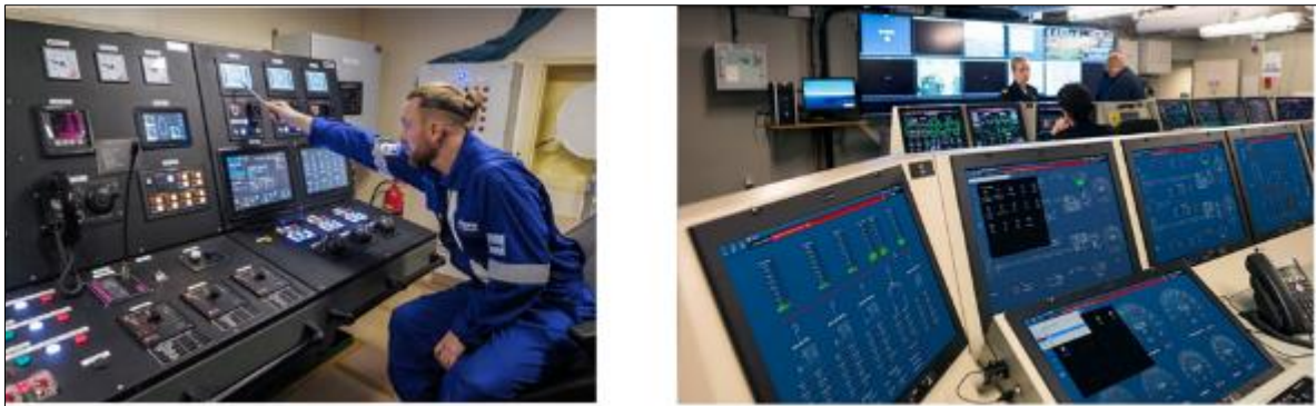
Figure 8 An IoT-Enabled Automation and Control Centre
